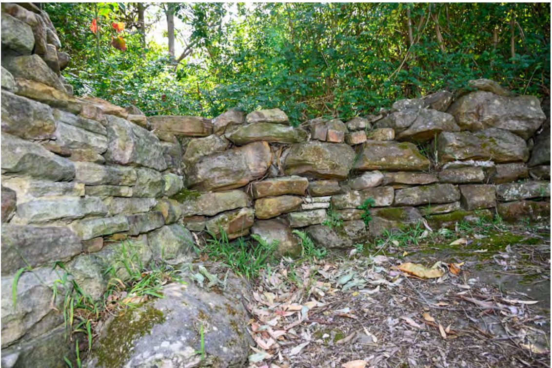
Southern property boundary. Heading east towards St Vincents Road. Common boundary with 53 Gore Street.
