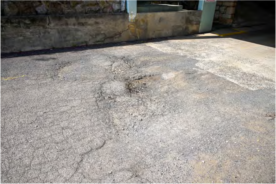
Internal access road from River Road. Heading south through the 'tunnel'. Damaged road paving.
