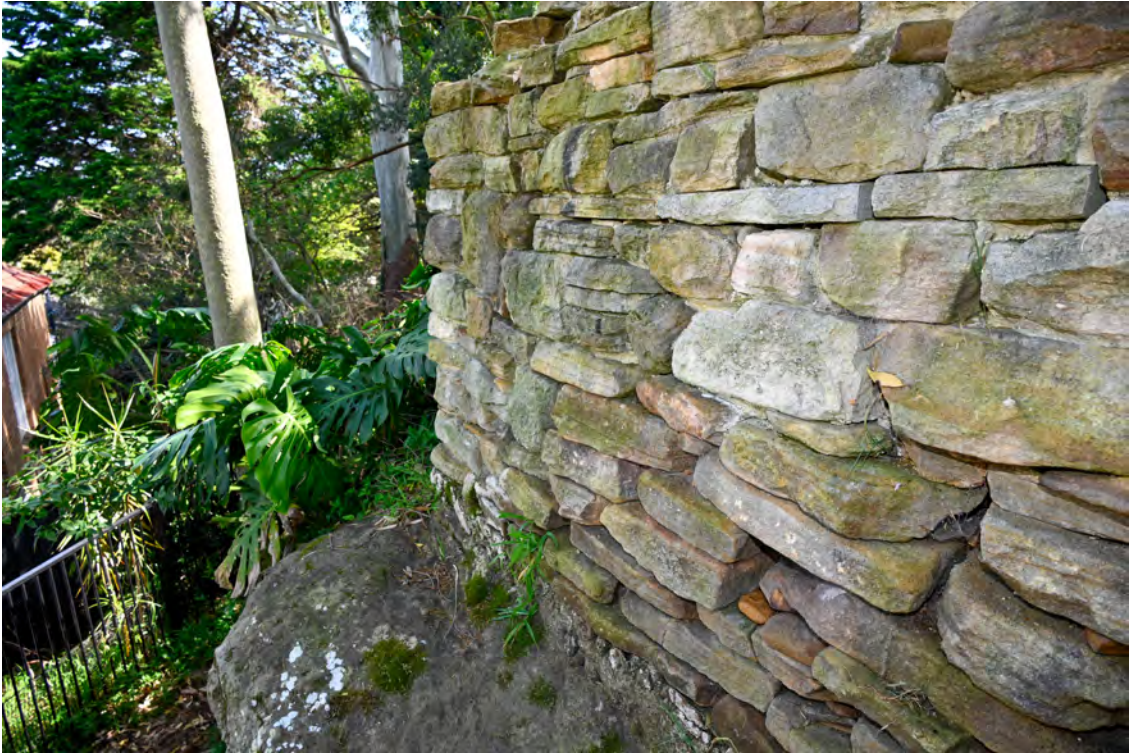
Southern property boundary. Heading east towards St Vincents Road. Common boundary with 53 Gore Street.
