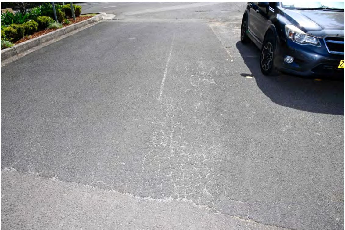
River Road. Area of the proposed substation works. Adjacent internal access road. Heading north towards River Road. Cracked and crazed road paving.
