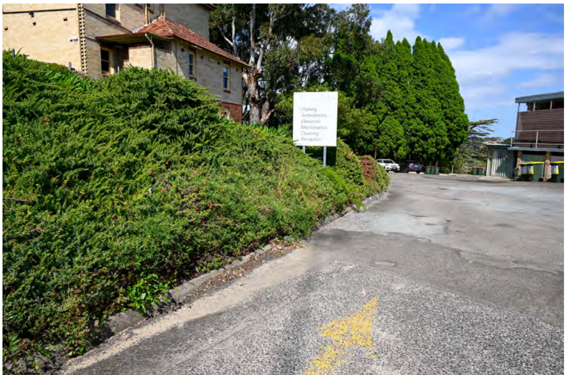
Internal access road. Heading south. Area of 'Service and deliveries'. Retaining structure below the area of road works.
