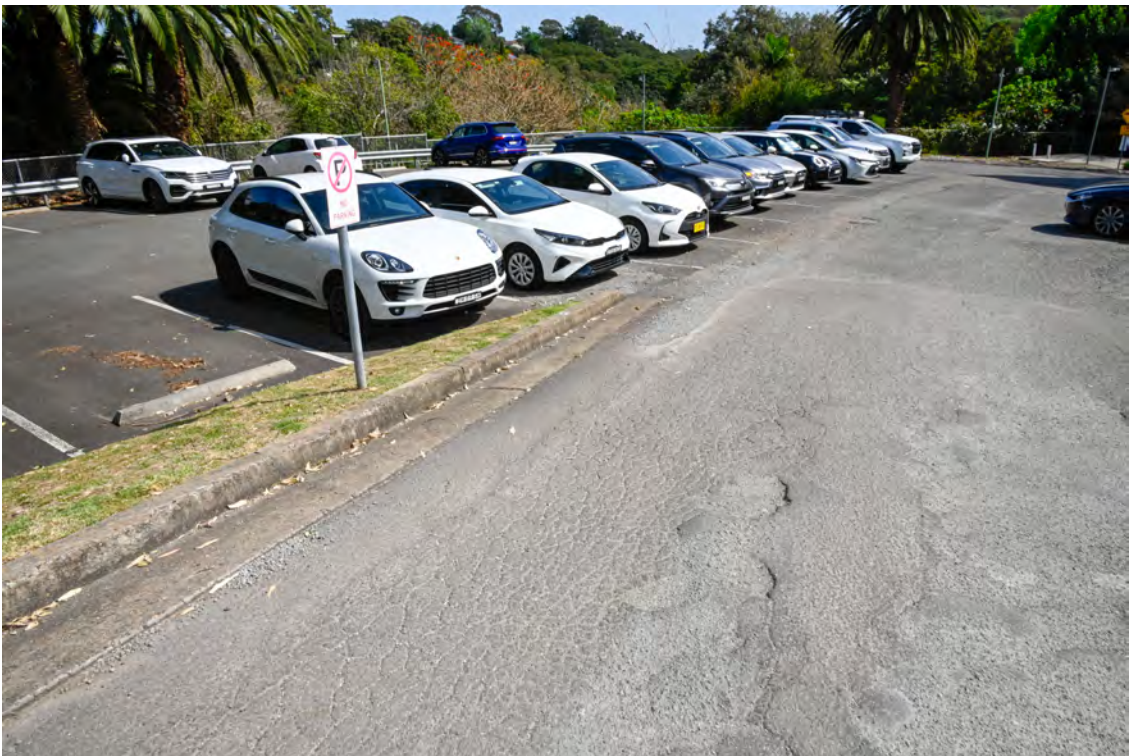
Western side of the property. Internal access road. Heading north towards River Road. Damaged road paving.
