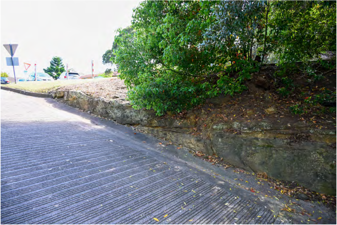
Hospital access road from St Vincents Road. Heading west / uphill towards Pallister House. Rock face on the northern side of the road.
