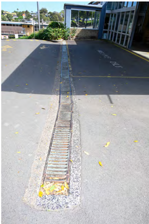
Internal road between Pallister House and 'Ambulatory Services'. Heading south-west. Strip drain.
