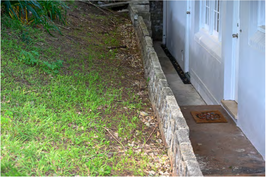
Southern property boundary. Heading east towards St Vincents Road. Common boundary with 24 Gore Street.
