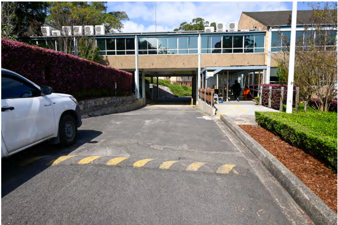
Internal access road from River Road. Heading south approaching the overhead walkway. Damaged road paving.
