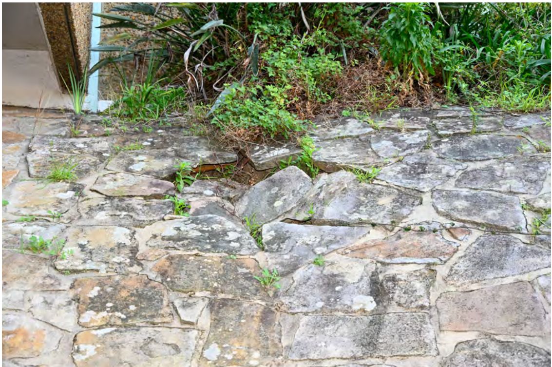
Internal access road from River Road. Heading south. Area of 'Service and deliveries'. Collapsed section of the retaining structure.
