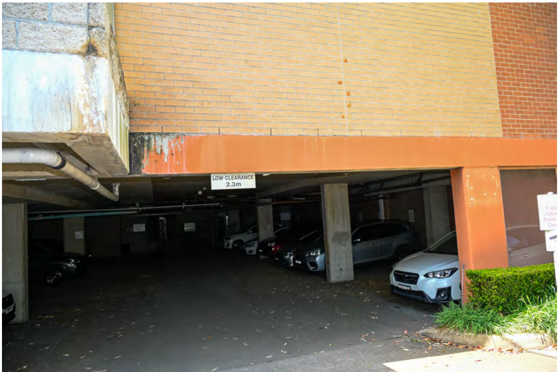
Western side of the property. Internal access road on the western side of the hospital building. Heading north towards River Road. Structure above the undercover parking.
