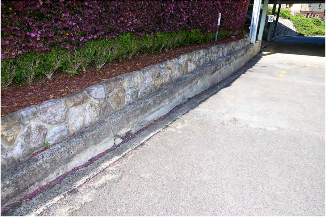
Internal access road from River Road. Heading south approaching the overhead walkway. Retaining wall.
