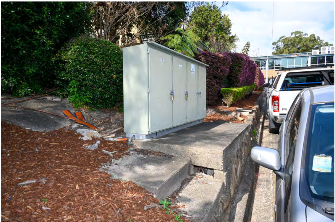
River Road. Area of the proposed substation works. Area on the eastern side of the internal access road. Existing electrical plant.
