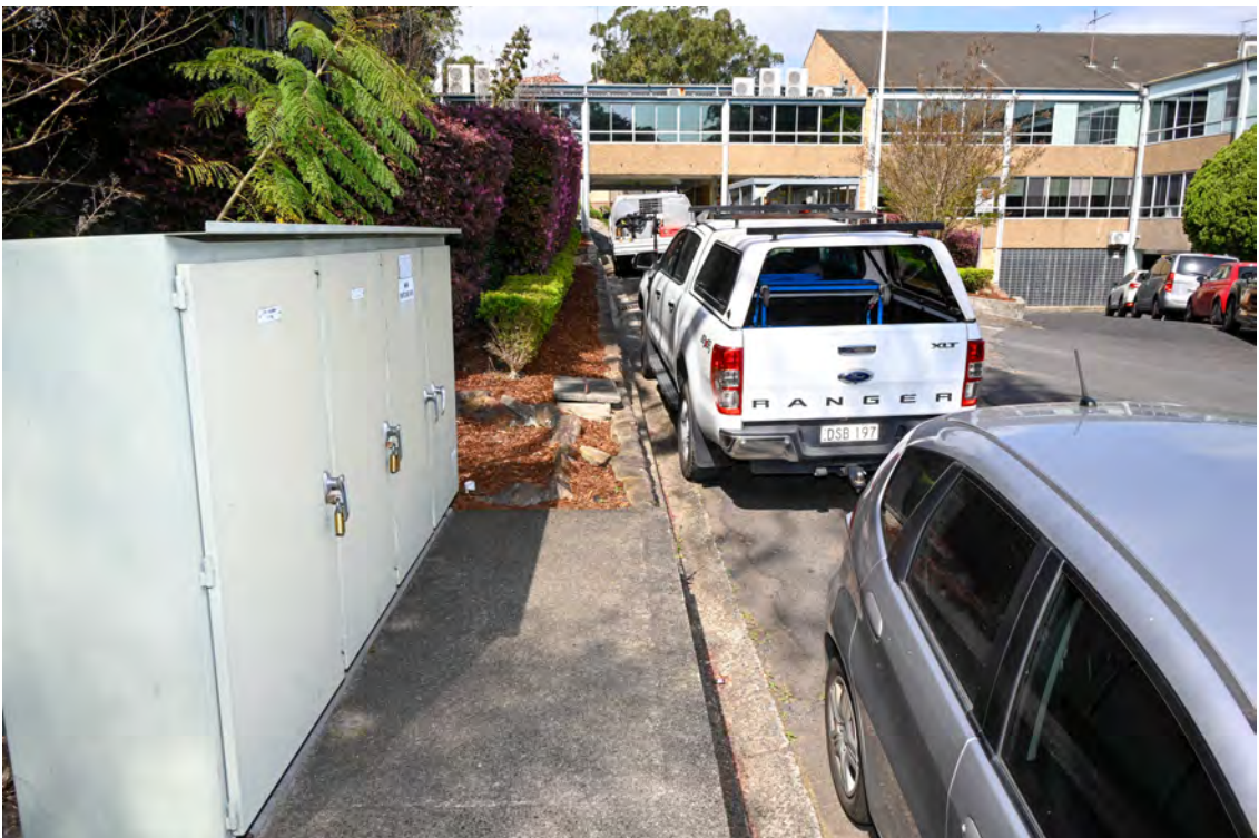
River Road. Area of the proposed substation works. Area on the eastern side of the internal access road. Heading south.
