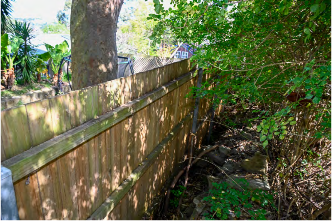
Southern property boundary. Heading east towards St Vincents Road. Common boundary with 51 Gore Street.
