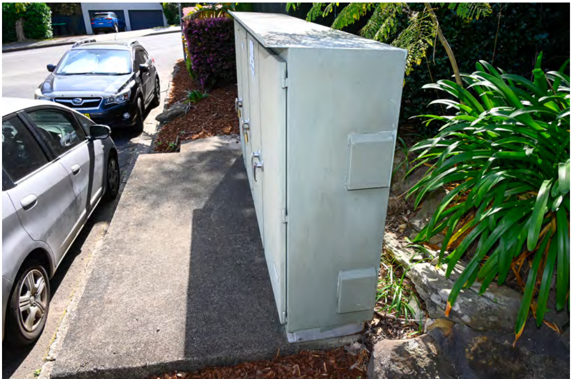
River Road. Area of the proposed substation works. Area on the eastern side of the internal access road. Record of the landscaping.
