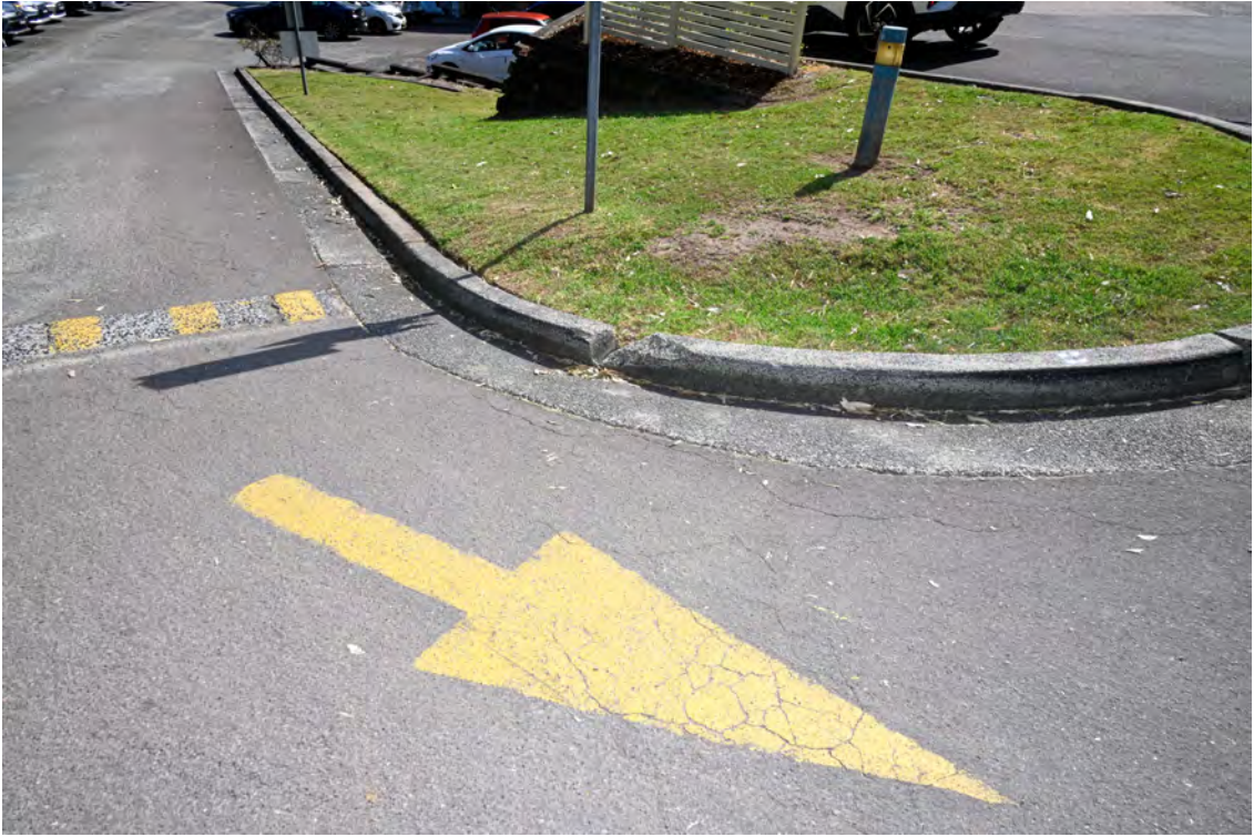
Western side of the property. Internal access road. Heading north towards River Road. Damaged kerb.
