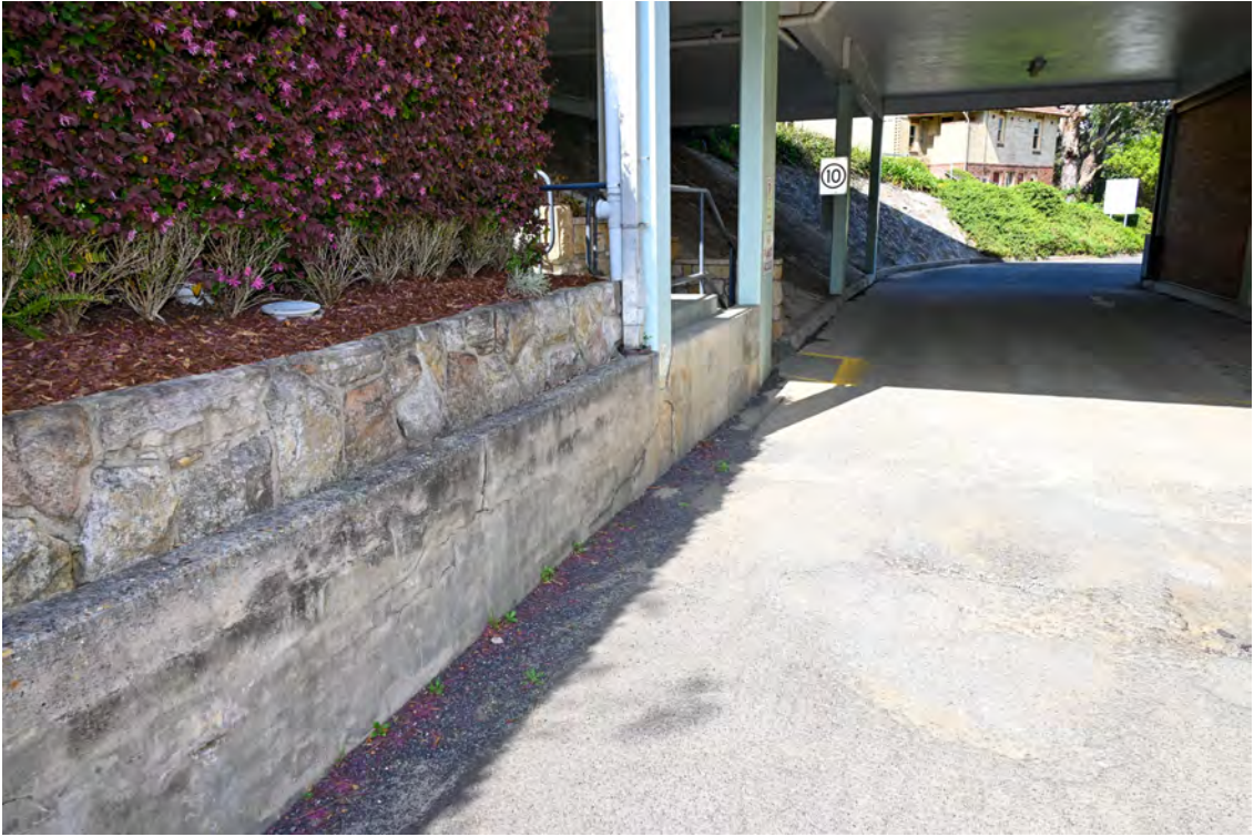
Internal access road from River Road. Heading south – overhead walkway. Retaining wall.
