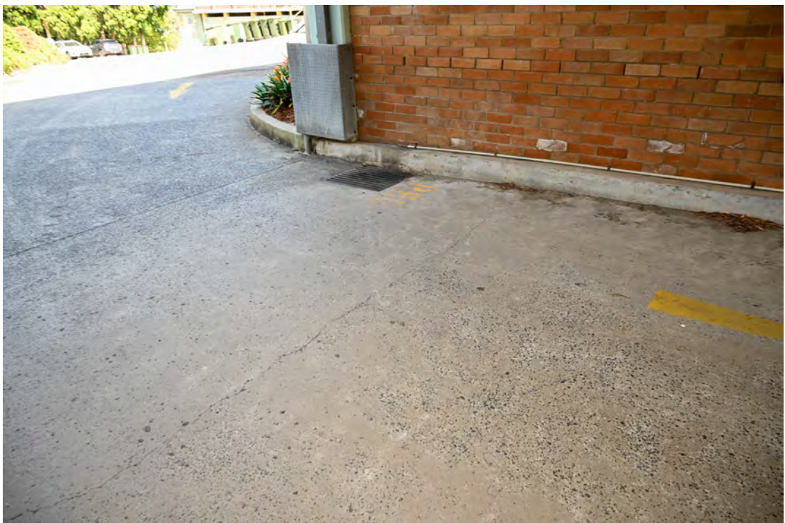
Internal access road from River Road. Heading south through the 'tunnel'. Cracked paving.
