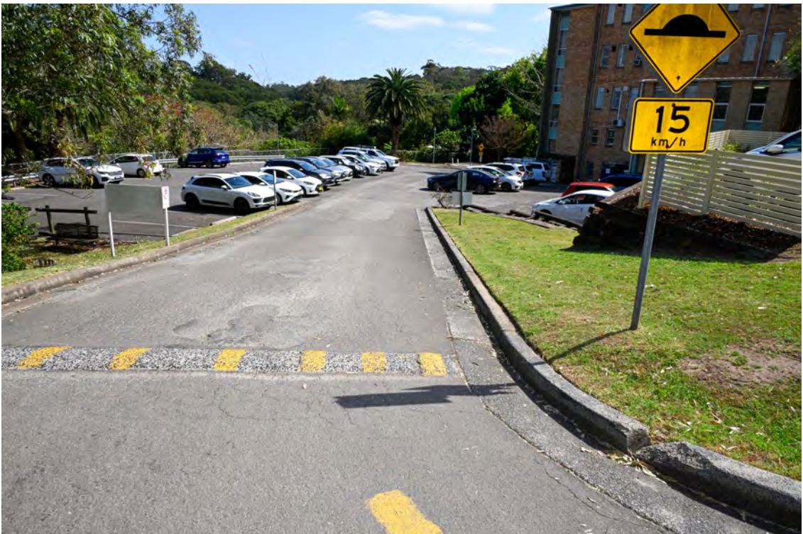
Western side of the property. Internal access road. Heading north towards River Road. Damaged road paving.
