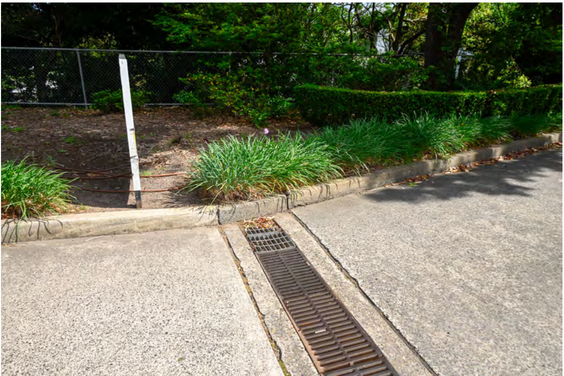
Western side of the property. Internal access road on the western side of the hospital building. Heading north towards River Road. Strip drain.
