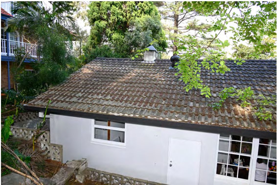
Southern property boundary. Heading east towards St Vincents Road. Common boundary with 24 Gore Street.
