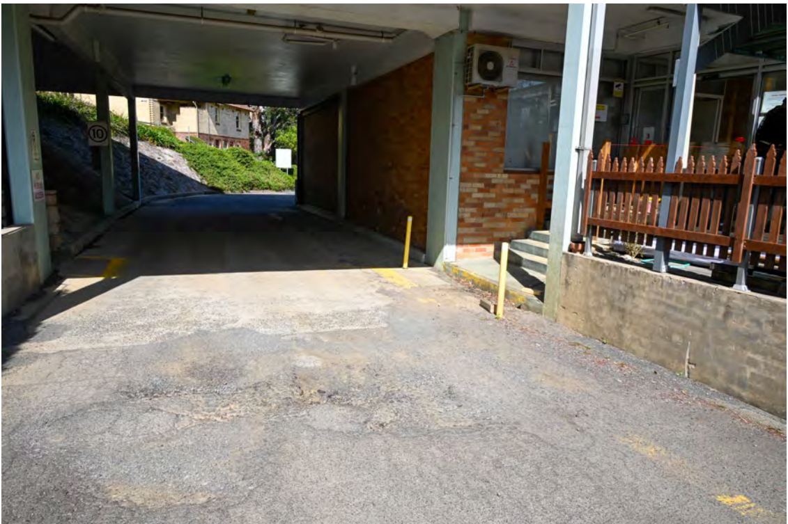
Internal access road from River Road. Heading south through the 'tunnel'. Damaged road paving.
