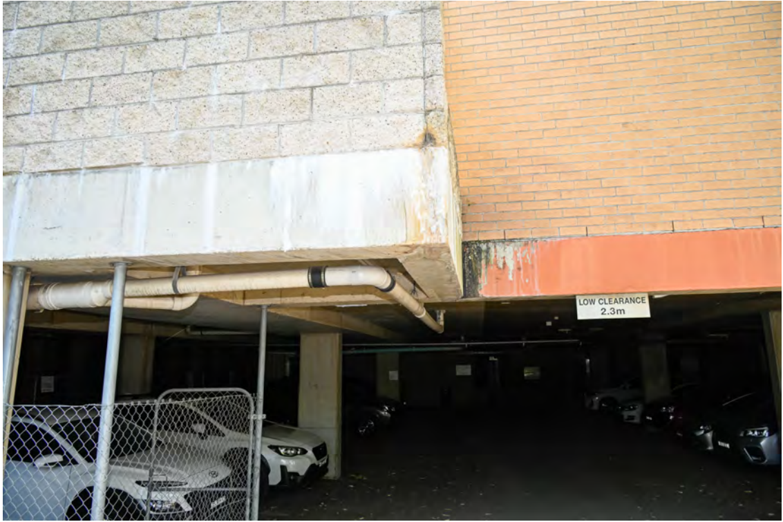
Western side of the property. Internal access road on the western side of the hospital building. Heading north towards River Road. Structure above the undercover parking.
