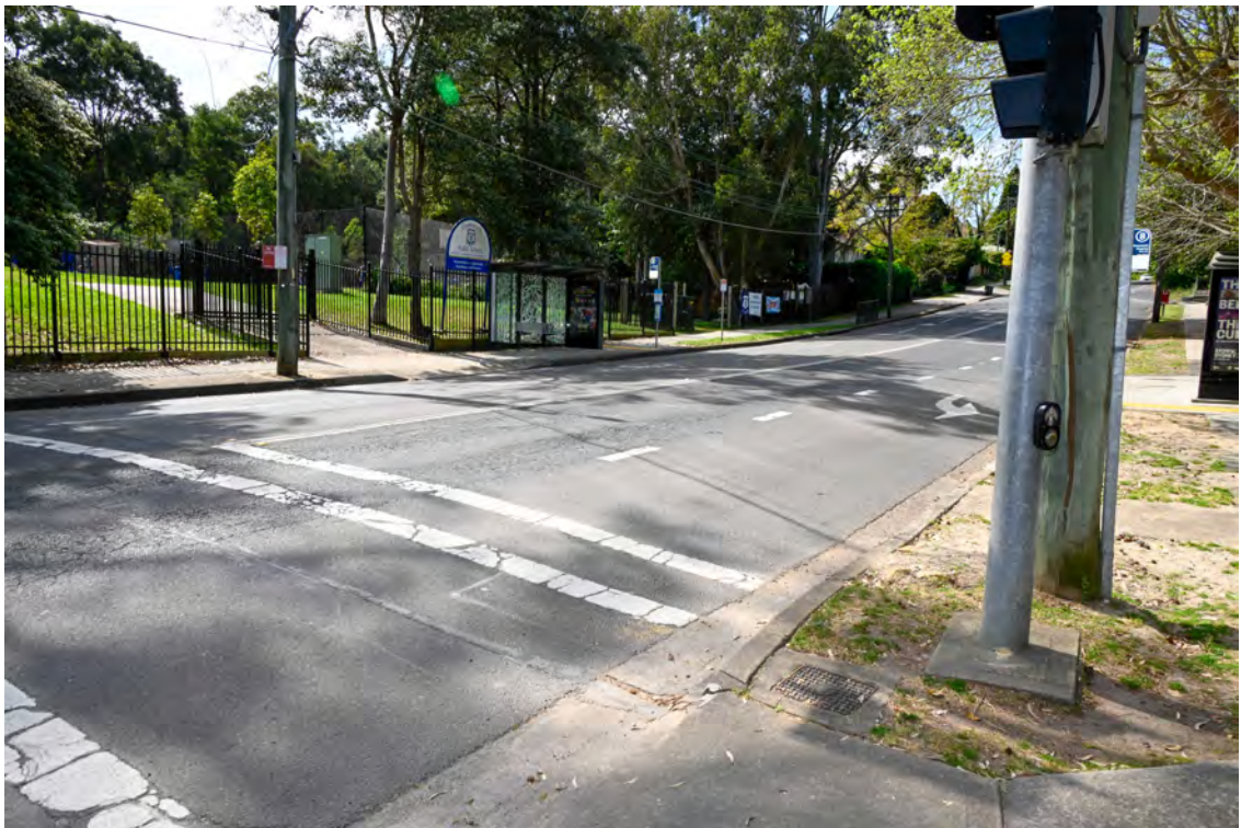
Internal access road on the western side of the hospital building. Intersection with River Road. Cracked and crazed road paving.
