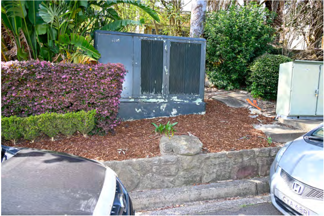
River Road. Area of the proposed substation works. Area on the eastern side of the internal access road. Electrical kiosk no. 2385.
