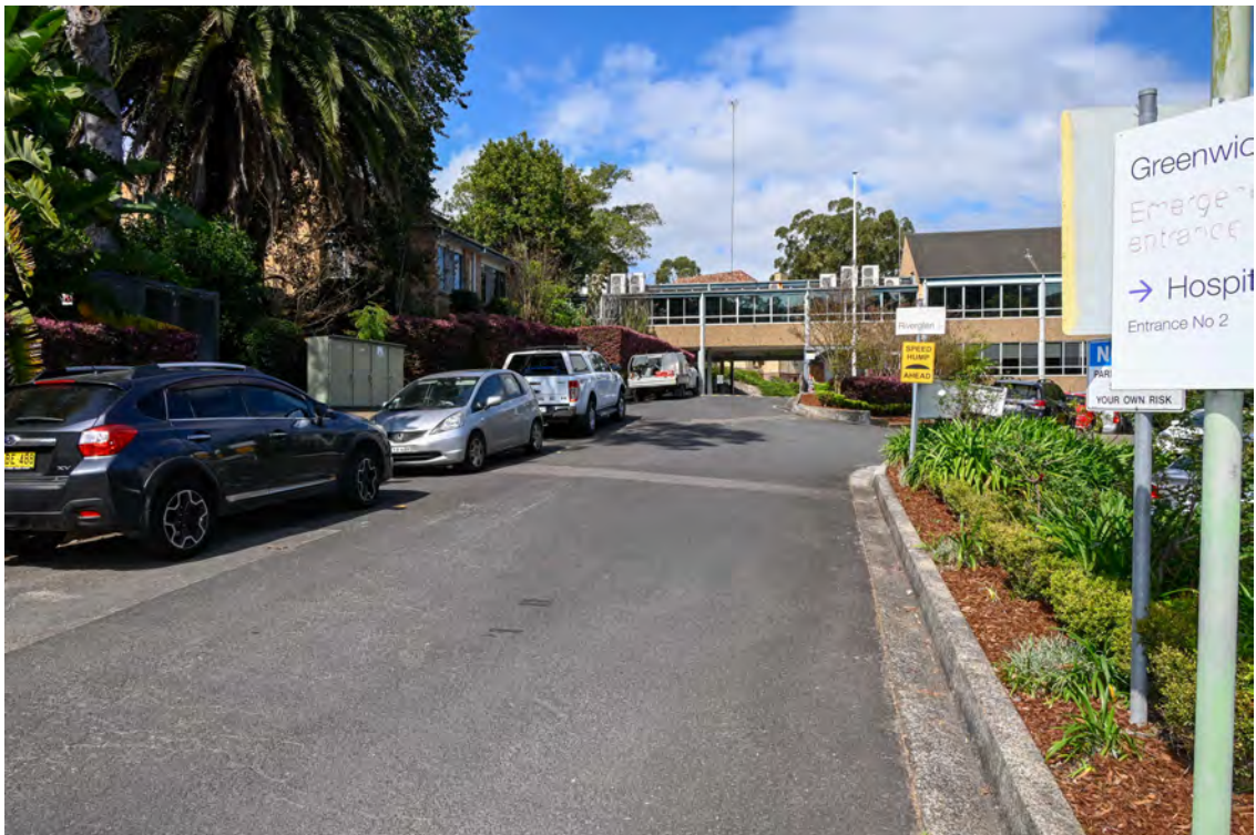
River Road. Area of the proposed substation works. Internal road. Heading south. Cracked and crazed road paving.
