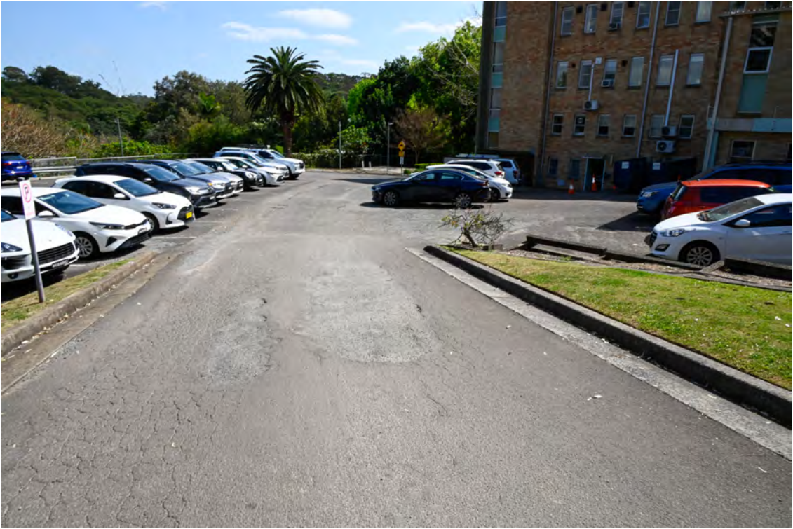
Western side of the property. Internal access road. Heading north towards River Road. Damaged road paving.
