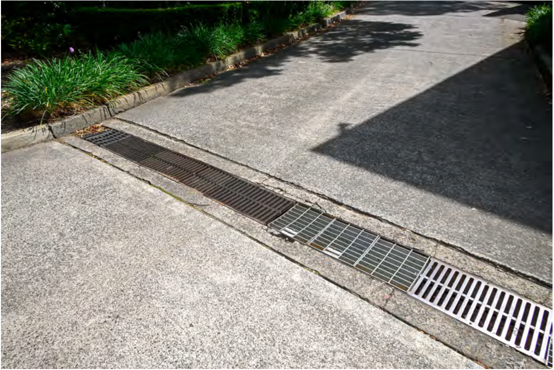
Western side of the property. Internal access road on the western side of the hospital building. Heading north towards River Road. Strip drain.
