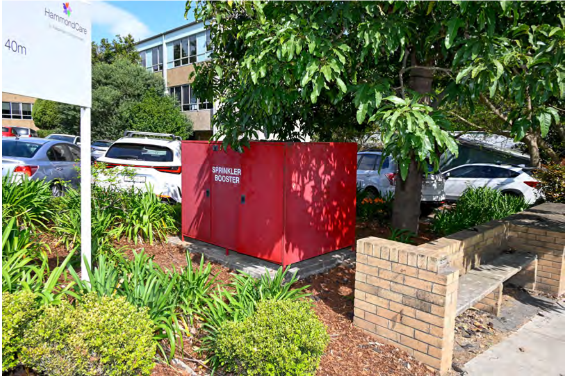
River Road. Area of the proposed substation works. Adjacent 'Sprinkler Booster' enclosure.
