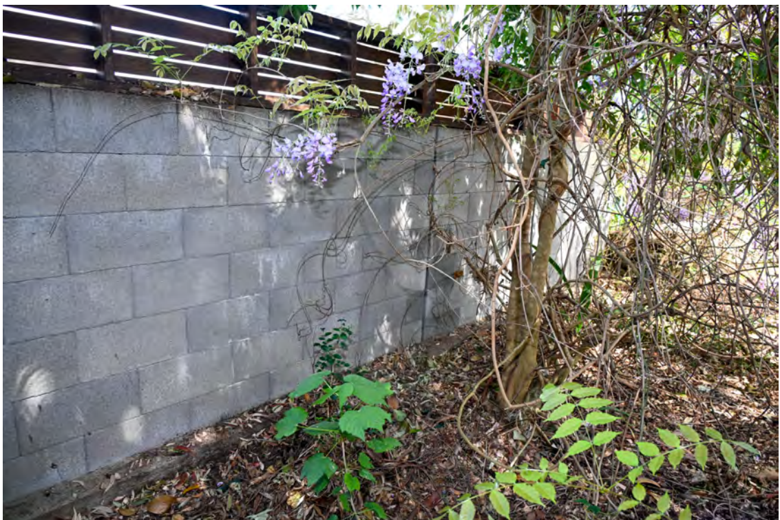
Southern property boundary. Heading east towards St Vincents Road. Common boundary with 51-47 Gore Street.
