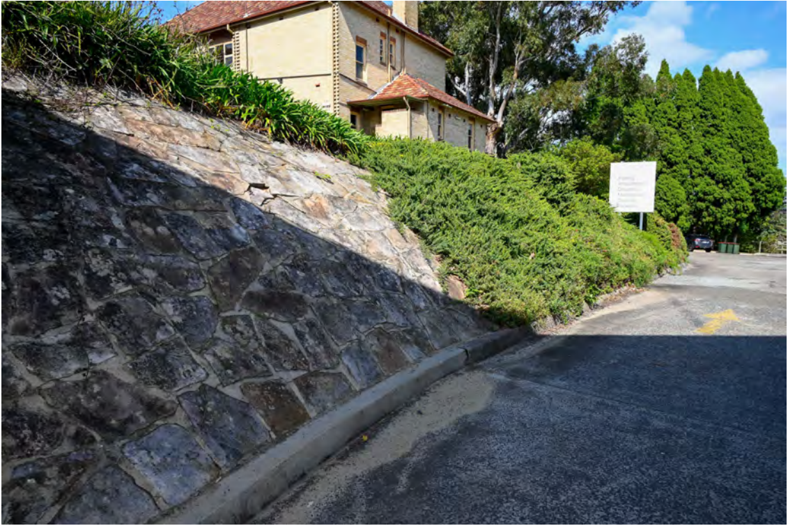
Internal access road from River Road. Heading south. Area of 'Service and deliveries'. Retaining structure.
