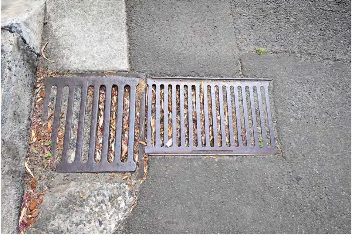
River Road. Area of the proposed substation works. Internal road. Heading south. Silted up strip drain.
